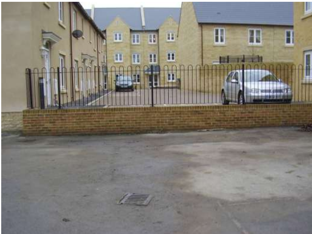
Area 6b Road gully, in low area behind houses along Bridge Street, with no apparent outfall except to seep into the ground below. Barrier caused by raising of Aquarius (14-12-08).
