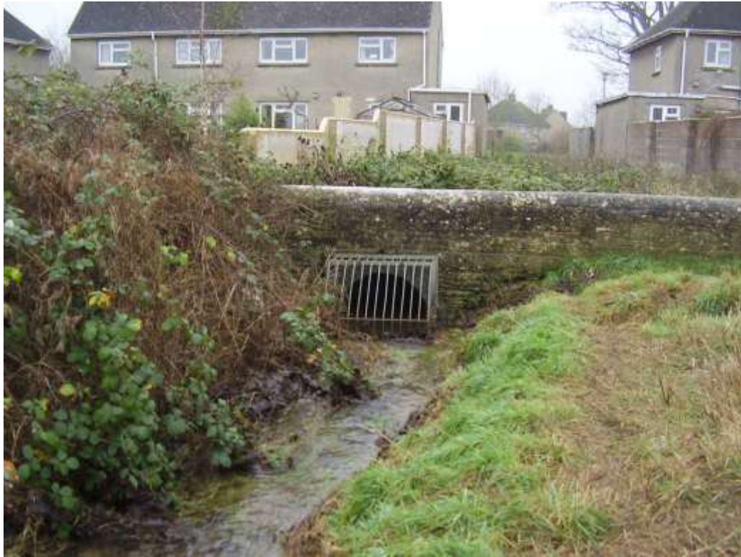
Area I – Eastfield Road and Hailey Road Inlet grille to Hailey Road Drain
