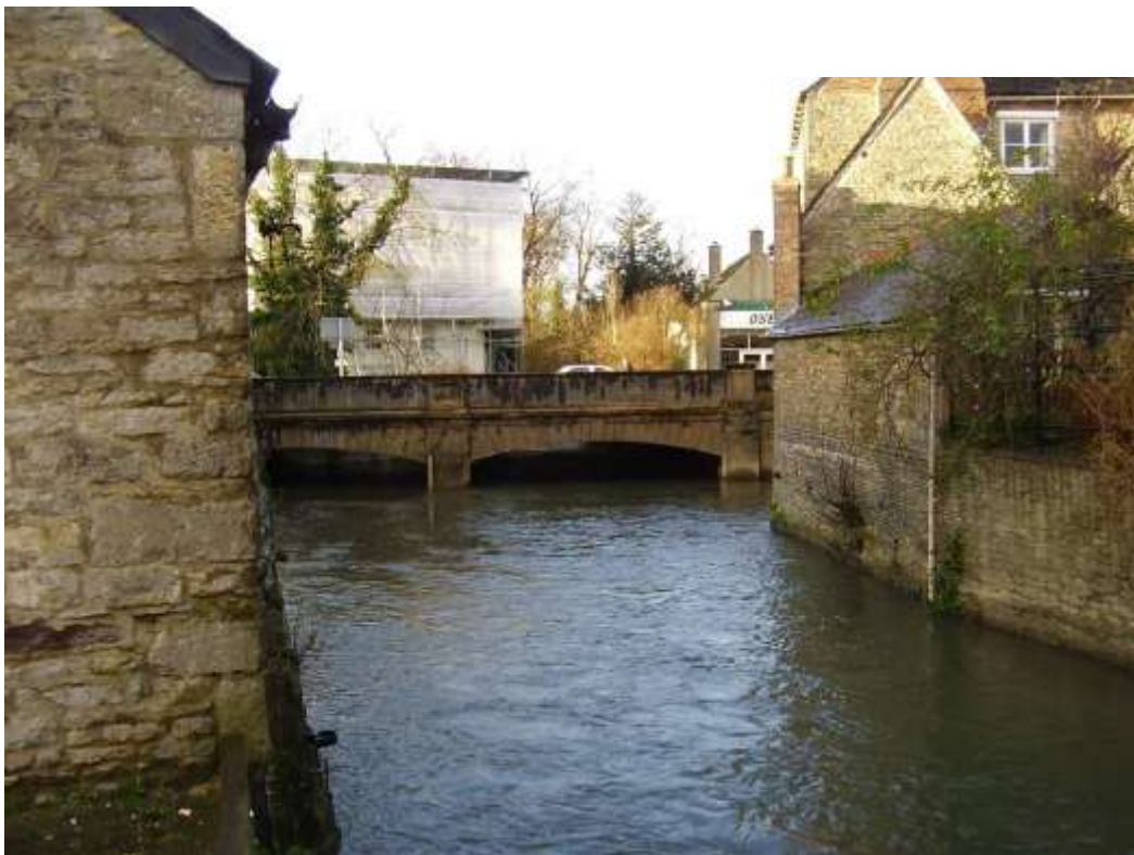
Area 6a View of downstream side of the bridge under Bridge Street
