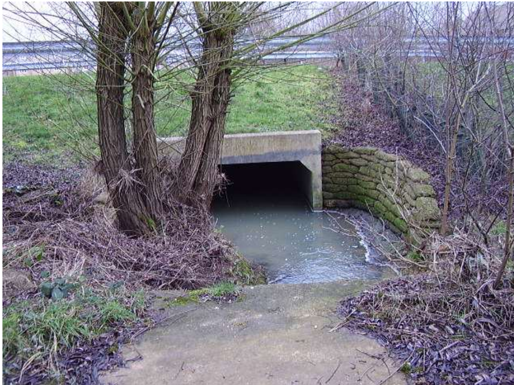
Area 5 – Madley Brook Upstream view of culvert C04 under Madley Way from top of low concrete bridge
