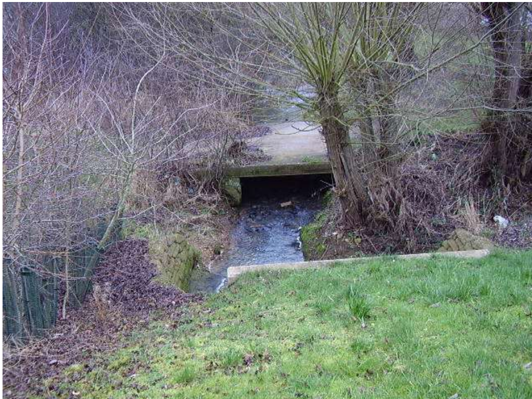
Area 5 – Madley Brook View of low concrete bridge upstream of culvert C04
