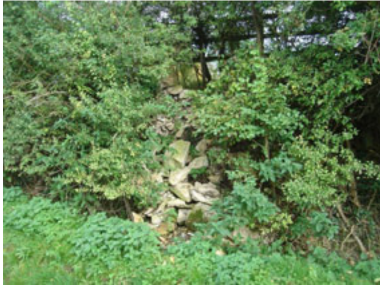
Area I – collapsed wall in ditch opposite The Old Farm
