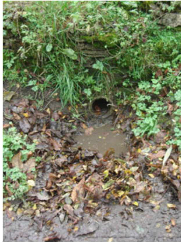
Area 3 – one of the culverts directing surface water from the highway into the watercourse
