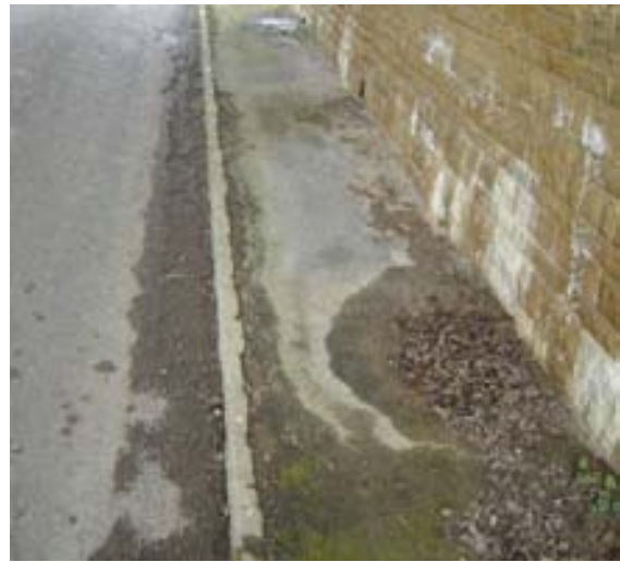
Area 5 - Flood damage under A361 Bridge
