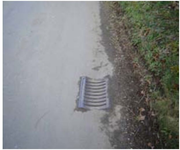
Area 3 - Highway drainage flood damage
