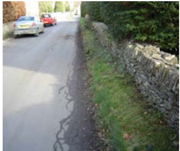
Area 3 - Highway drainage water damage at Filkins
