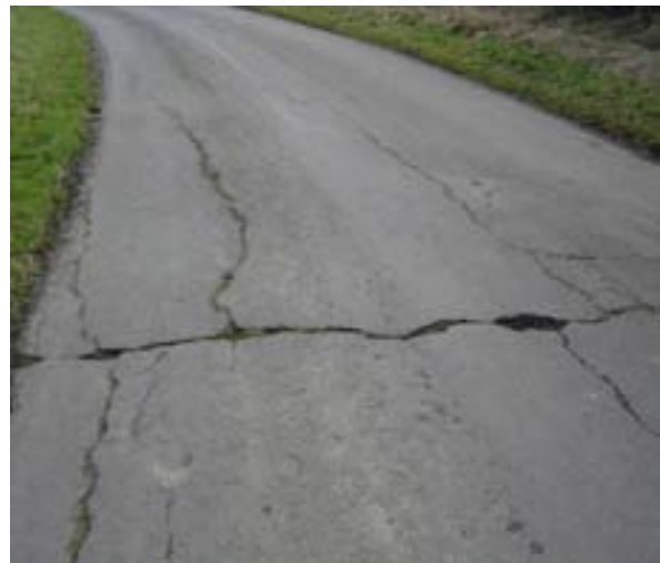
Area 5 - Flood damage at Little Barrington Road
