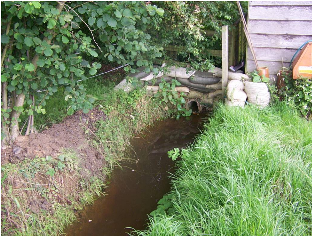
Photo 6 - The same ditch as seen in the previous photo showing the increase of water level which leads to surcharging of the pipe and flooding of property.
