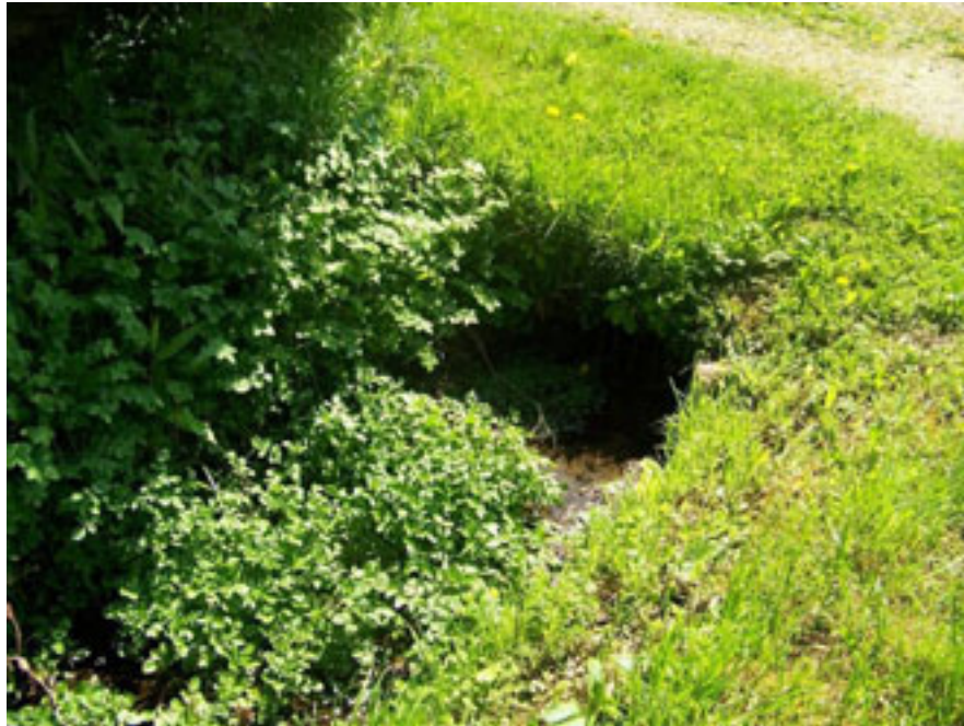
Photo 7 - Highway drainage on southern side of road above Station Road junction near Model Cottages. Channel was overgrown on inspection in May 2008.
