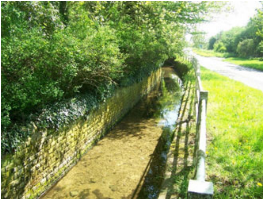
Photo 5 - Black Bourton Brook – looking downstream from Station Road Bridge. Channel capacity smaller than upstream of the bridge (Photo 4)
