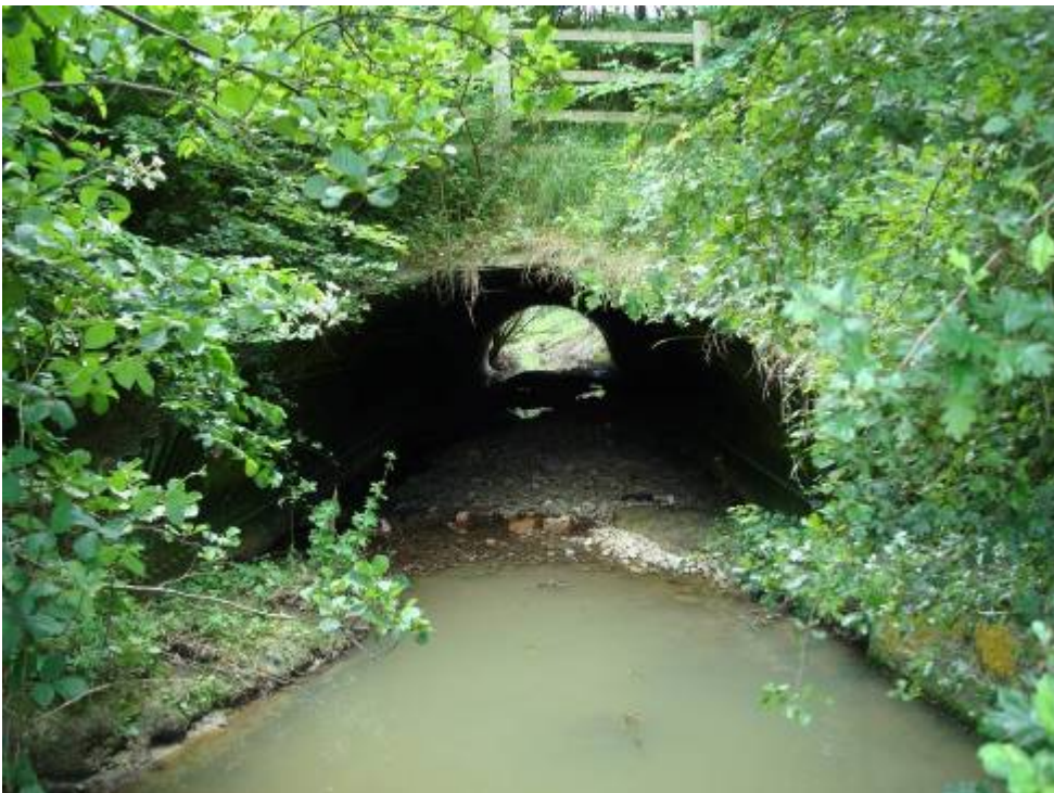
Photo 12 – New A40 crossing requiring maintenance of the channel bed (Chil Brook).
