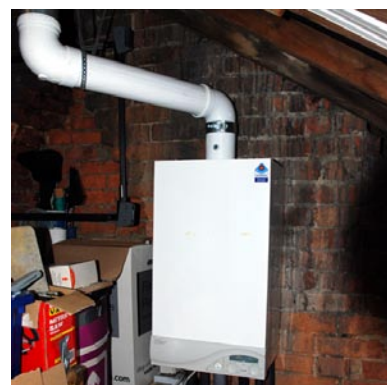
Fig. 20 Modern gas fired combi-condenser boiler
