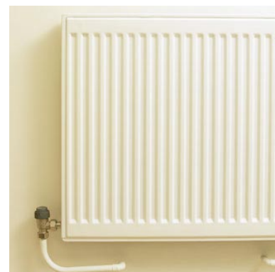
Fig. 25 Modern wall-mounted pressed steel radiator
