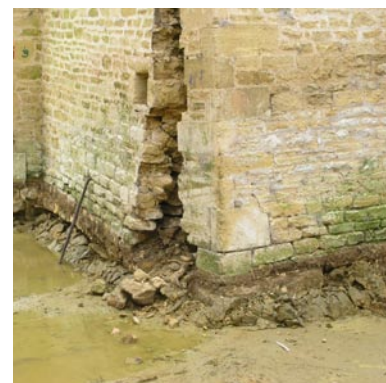
Fig. 16 Care must be taken not to undermine walls with shallow footings
