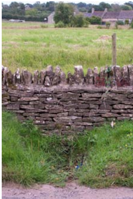
Photograph 18: Grip on Akeman Street. Weep holes required in dry stone wall to direct water to Combe Green.
