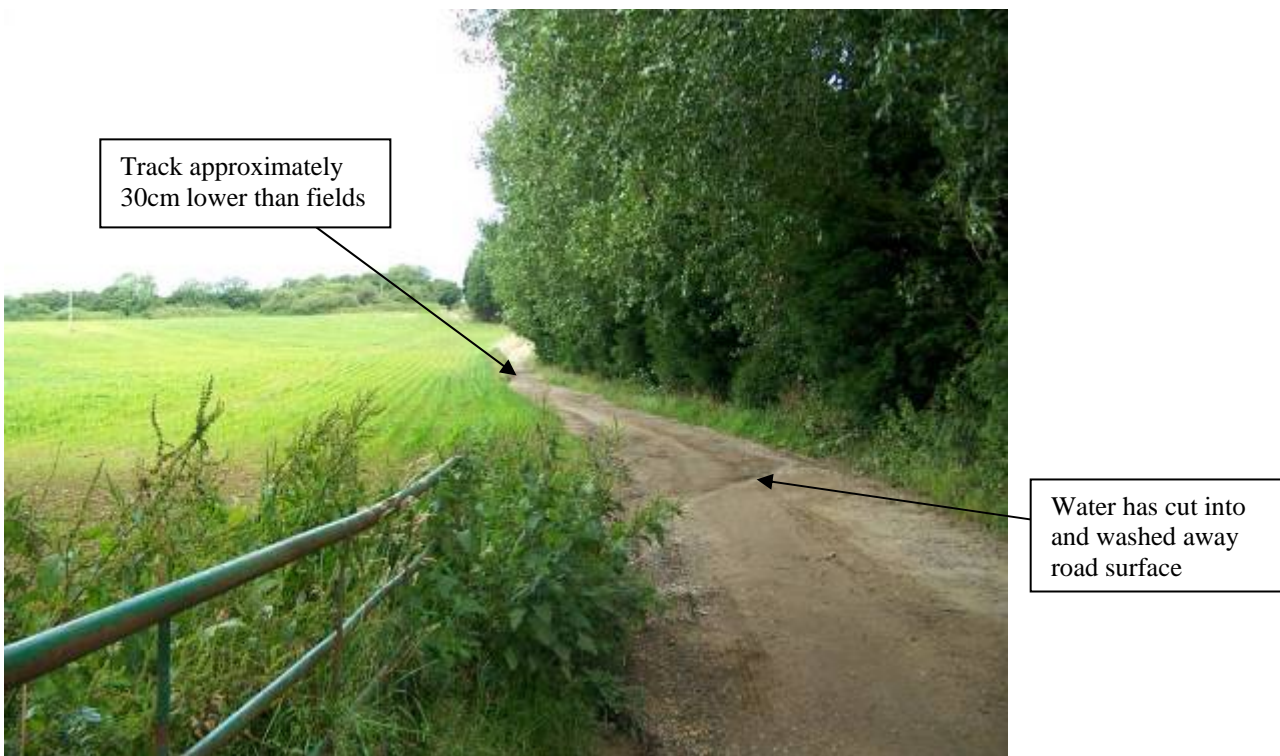
Photograph 11: Track off Golden Lane which water is channelled down
