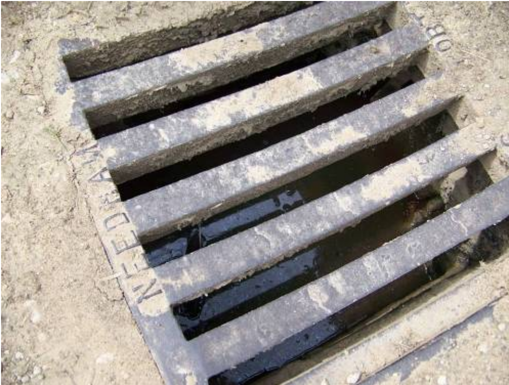
Photograph 10: Blocked drain on estate
