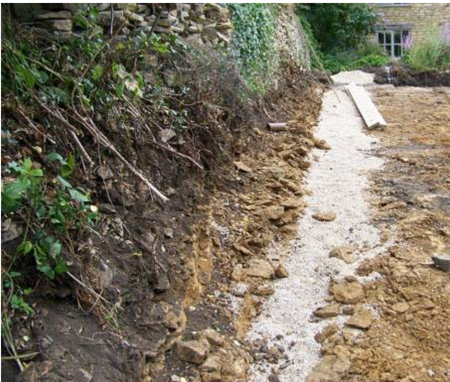
Photograph 26: Newly engineered watercourse. The 2 90 degree bends were removed, so that it now runs in a straight line behind the properties.
