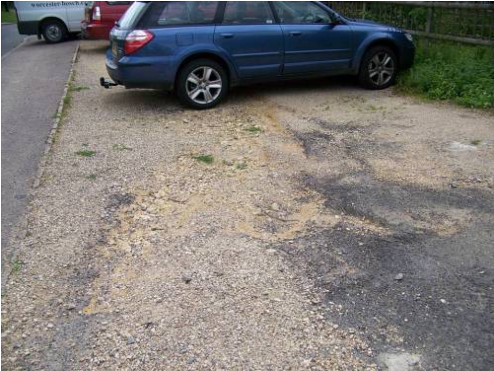
Photograph 19: Car Park at The Leys where water pools
