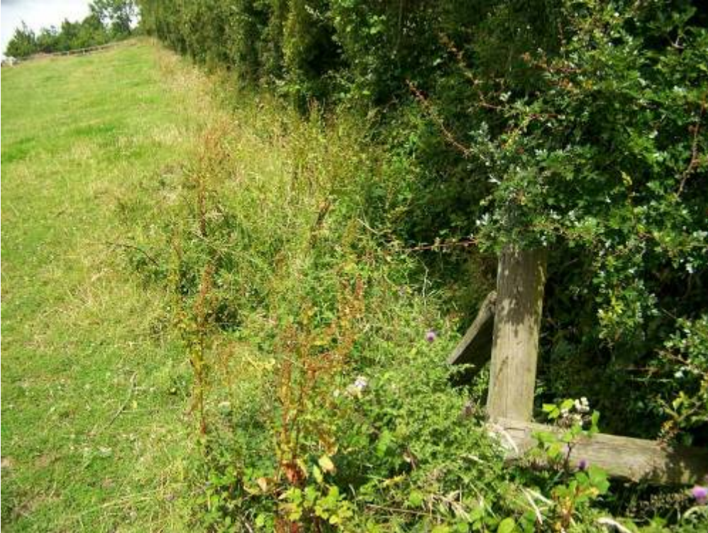
Photograph 22: Overgrown drainage ditch in field at the back of the Leys.
