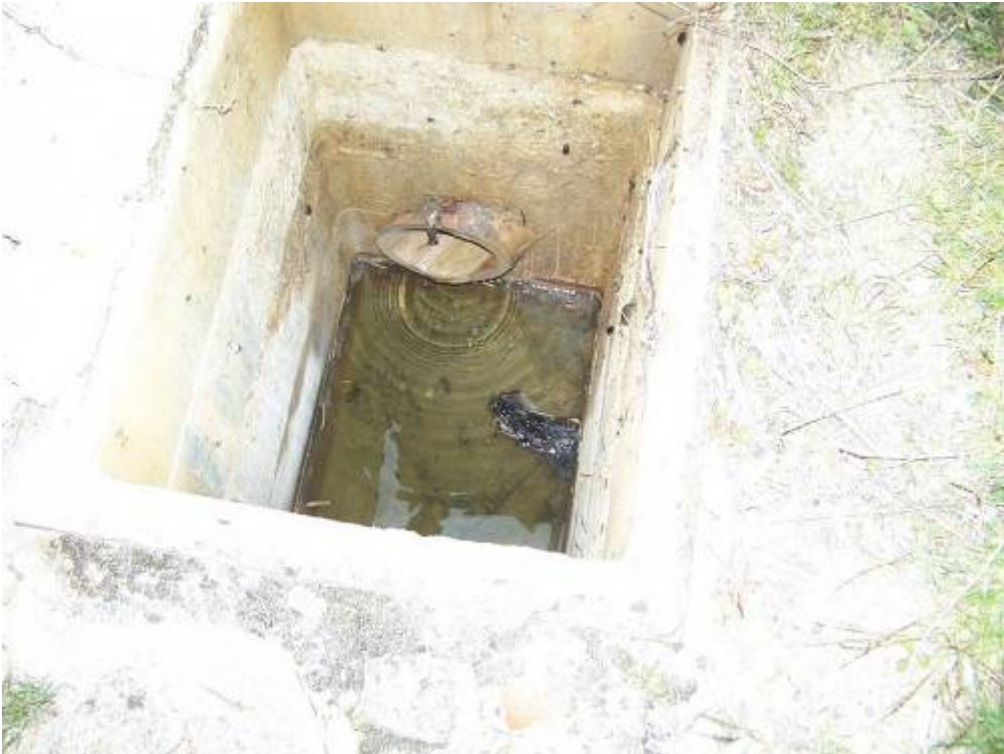
Photograph 18: Inspection Chamber in road by The Leys. In times of intense rainfall the cover is lifted due to the amount of water in the system.
