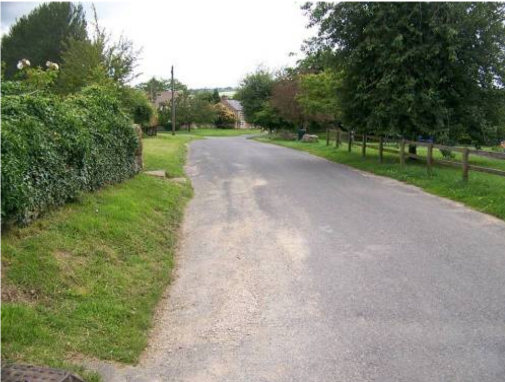
Photograph 16: Looking from the Leys towards the cross roads of Golden Lane and Roses Lane. Water is channelled along the road. There is no road drainage.
