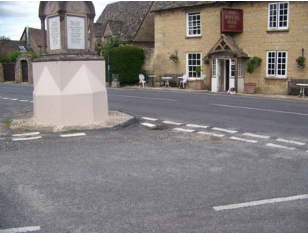
Akeman Street junction with war memorial – ponding occurred here July 07
