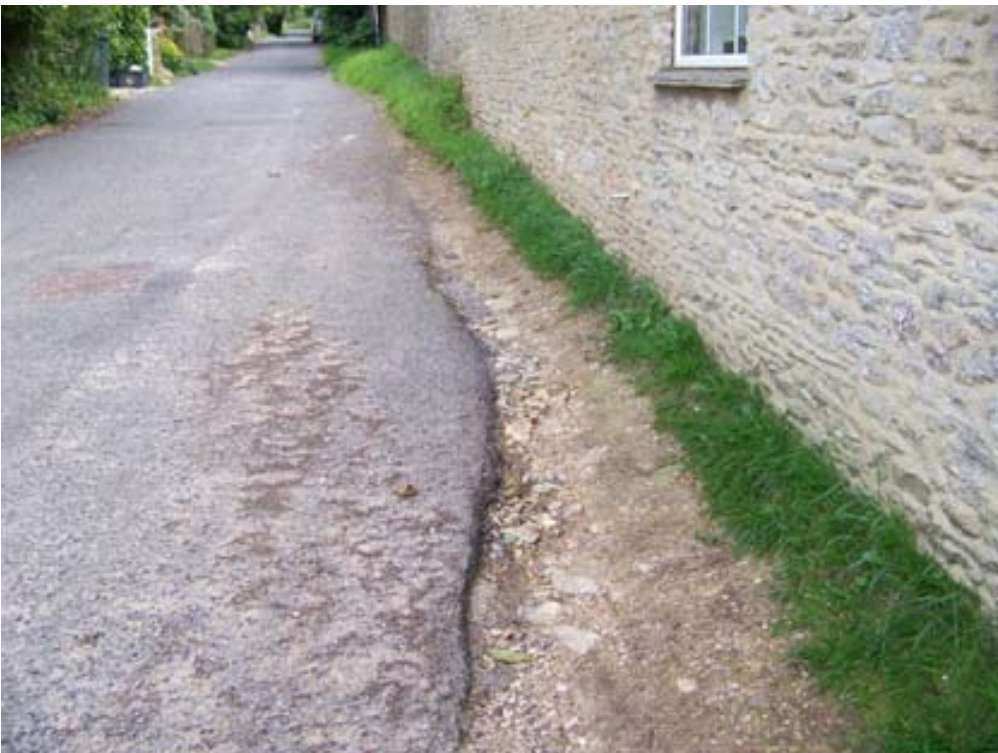
Flooding scour down Wilcote Lane – due to lack of highway drainage and run-off from land
