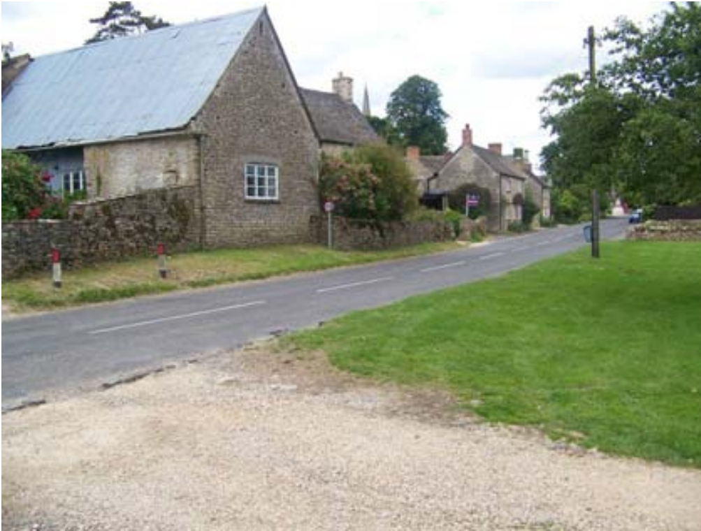
Lower End road – sloping drive down to properties and damaged kerbstones
