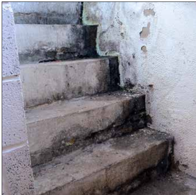
Fig. 9 Water damage to cellar steps in a Listed Building are often severe damp and condensation.
