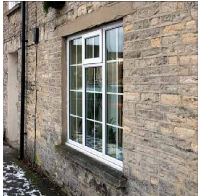
Fig. 8 Visually harmful double-glazing
