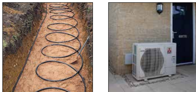
Fig. 12 Ground source pipework and air source heat pump
