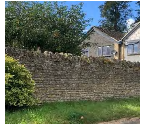
Significant Boundary Walls Remaining dry stone walls in various locations in the Character Area as identified in this Code Analysis. A significant feature in Cassington.
